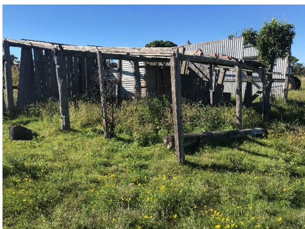
Looking northeast at the dilapidated cattle yards that have been constructed with timber and corrugated steel sheeting
